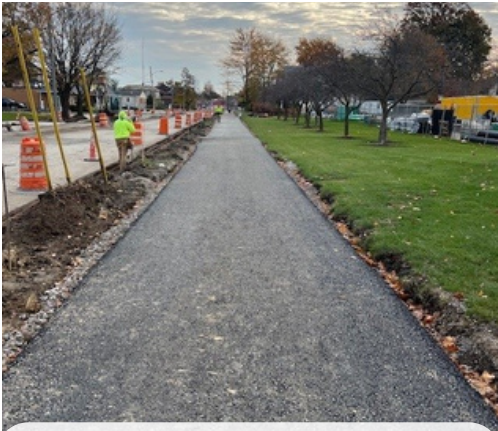
Creation of the East Broad Street shared-use path. Photo courtesy of City of Elyria.
