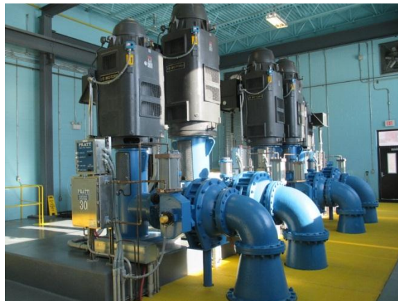
INSIDE THE NEW PUMP HOUSE: HIGH SERVICE PUMPS THESE ARE THE PUMPS THAT PUMP WATER TO THE MAINS
